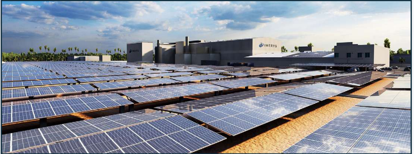
4.7 MWp solar plant at the Imerys-Zayani white-fused alumina plant
